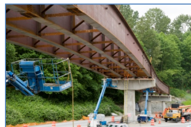
New HOV ramps being constructed to connect Highway 1 traffic to Grandview Highway at an improved Boundary Road intersection.
