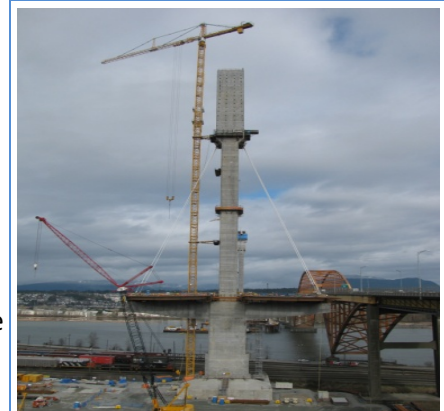
The first support cables for the main span of the Port Mann Bridge.
