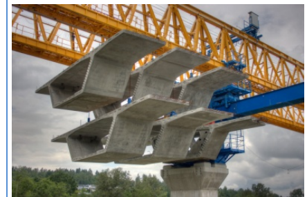
New bridge deck sections being held in place by gantry. The south approach of the new Port Mann Bridge is complete and the gantry is positioned over the north approach.
