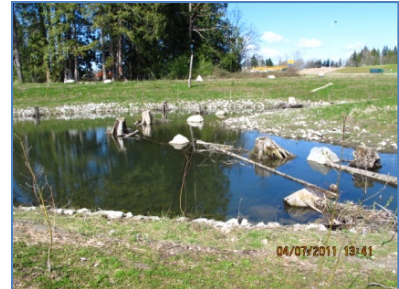
Hjorth Creek environmental enhancement work is now complete. The project is intended to maintain and enhance existing wildlife features.
